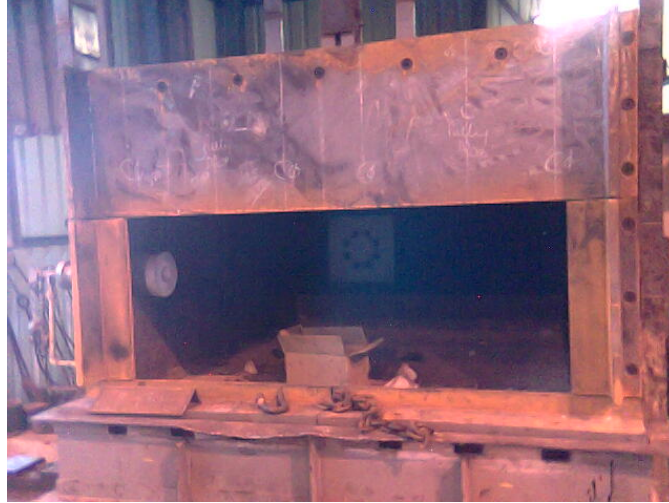
Fig 1: No 8 Furnace (Showing castings)
